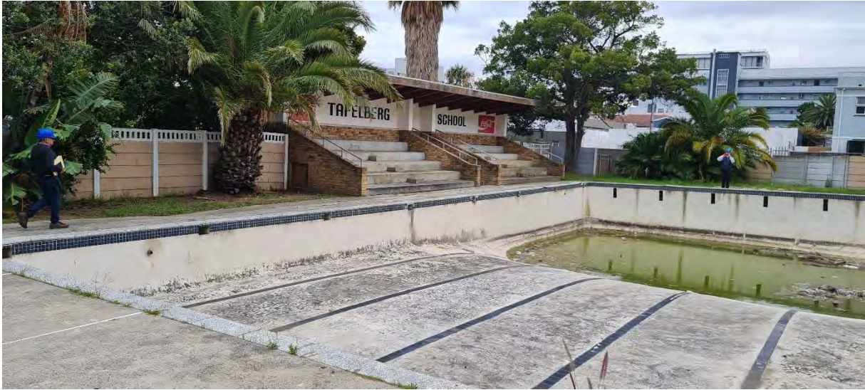
Figure 20: Abandoned Swimming Pool on the Land Portion Earmarked for Development
