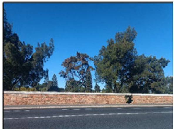
Figure 12. Degraded cemetery wall (captured 08/05/2024)
