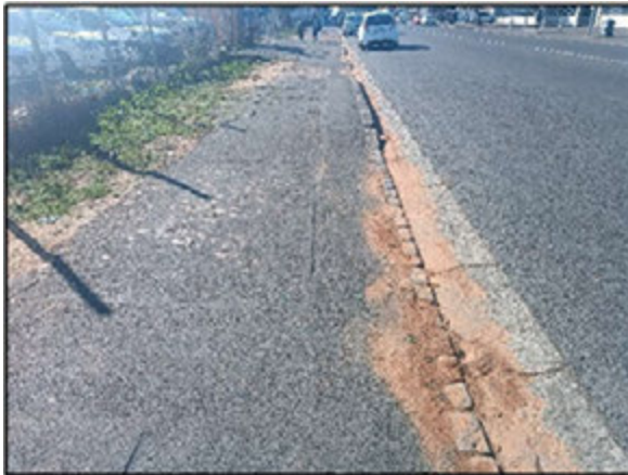
Figure 9. Degraded road infrastructure (captured 08/05/2024)
